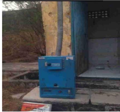
Incinerator not functional
