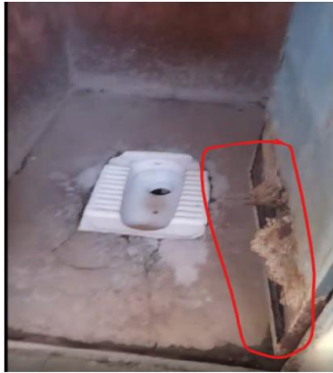
Door was broken
