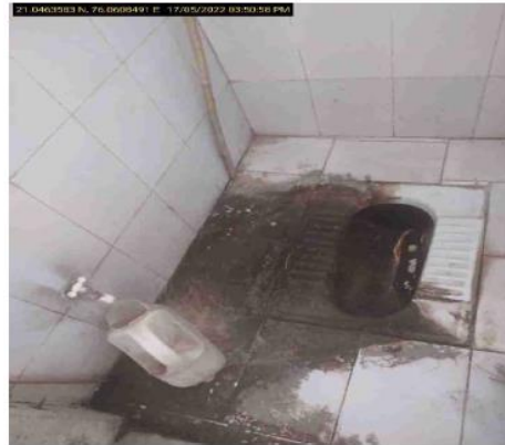
Toilet is not clean
