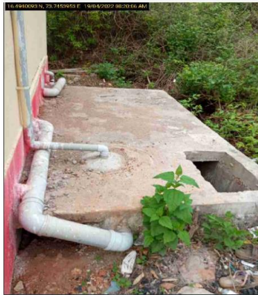
Safe disposal system not functional
