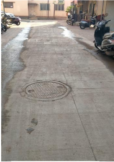
Settled sewer network at Bhor
