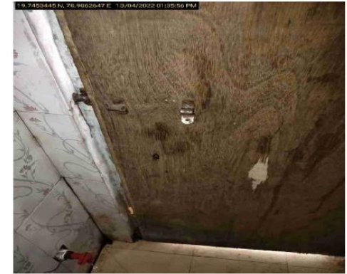
Bolting Arrangements was not Functional
